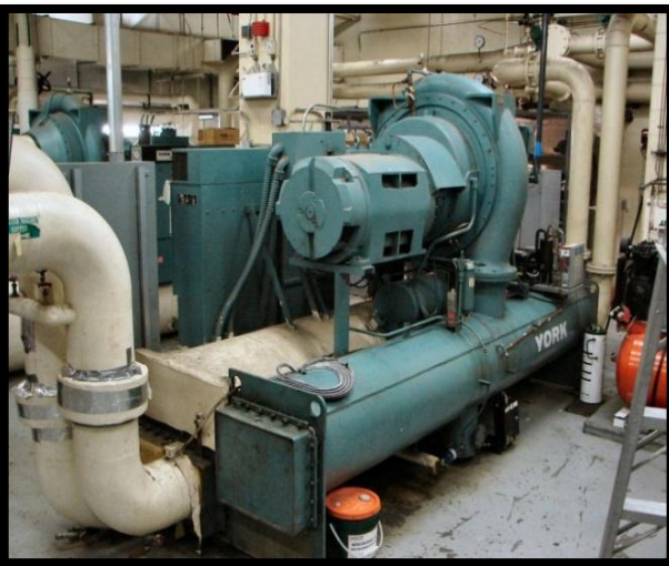
2 T Water Chilling Unit
