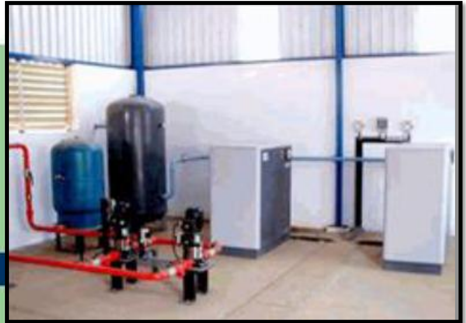
Compressed Air System
