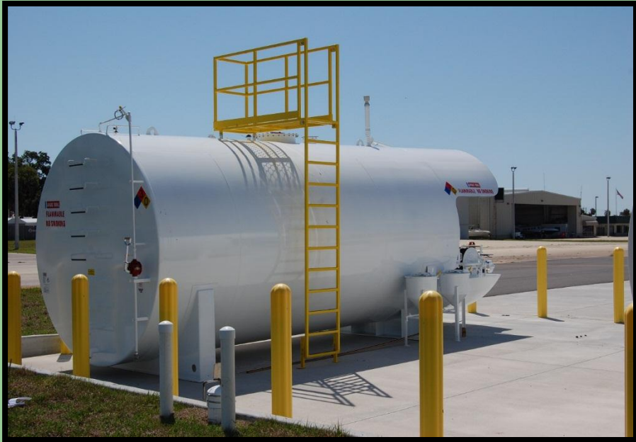
Fuel Storage Tank
