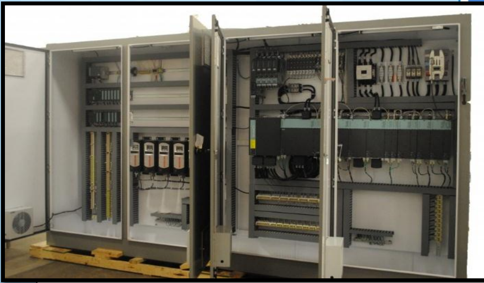
Electric Control Cabinet
