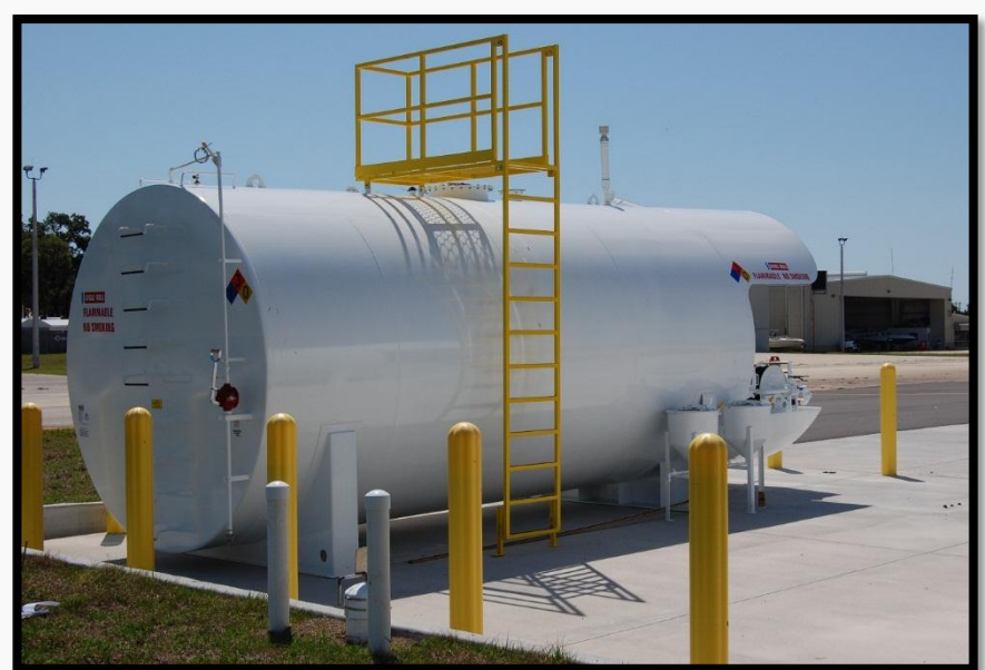
Fuel Storage Tank
