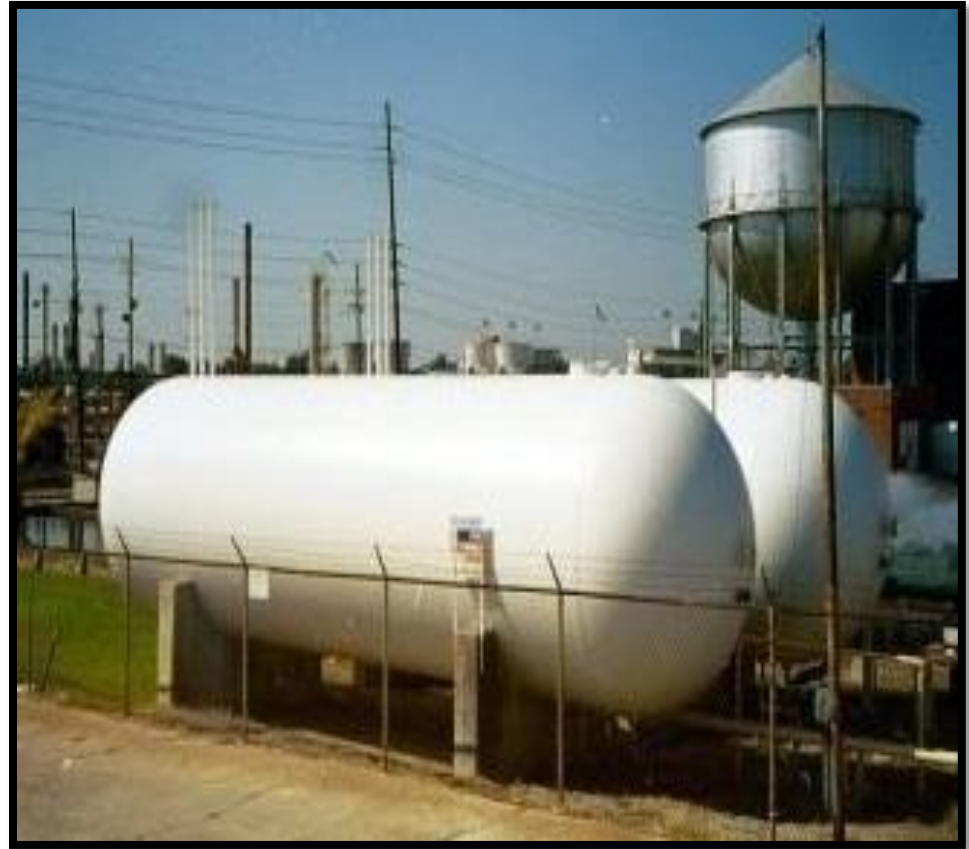
Chlorine Gas Storage Cylinder
